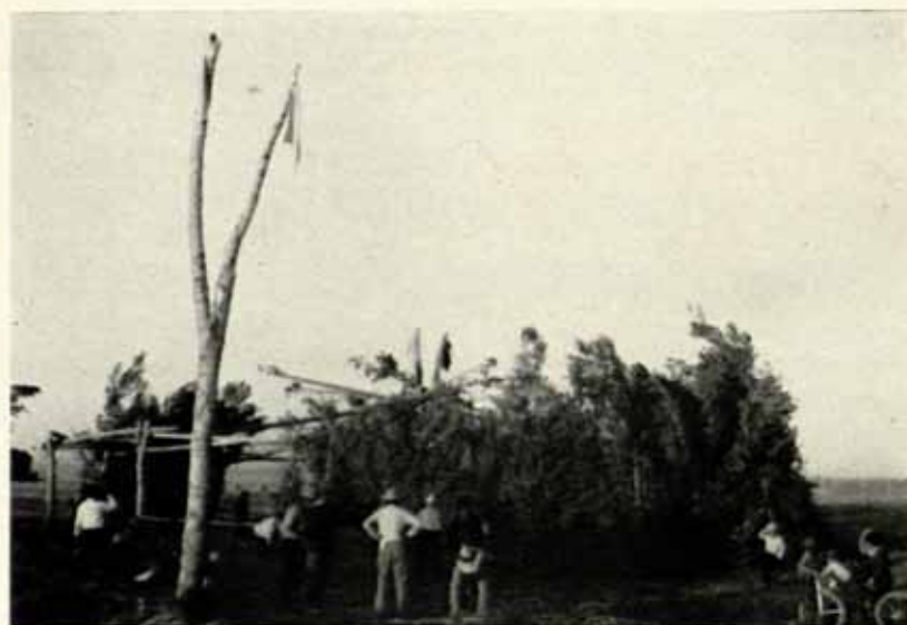
Upper: Men putting up the side roof poles, July 3, 1937, 6:50 p. m. Lower: The brush wall being finished, July 3, 1937, 7:30 p. m.
